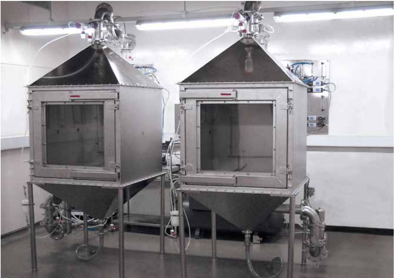
Whole Body Units with aerosol conditioning and exhaust air line – in the background a mounting panel with flow control units
